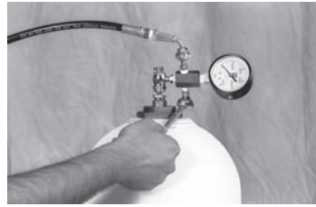
8. Open the bleed valve to bleed of nitrogen in the hose. Disconnect the charging assembly from the accumulator and the gas bottle.
